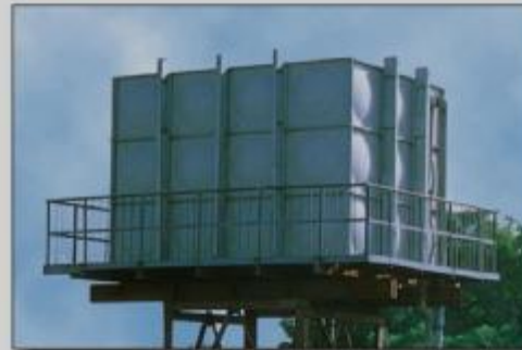
3m. Deep 36 KL tank for Drinking water at a Metro Colony.
