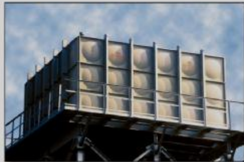
3m. Deep 108 KL tank for Drinking Water at a Housing Colony
