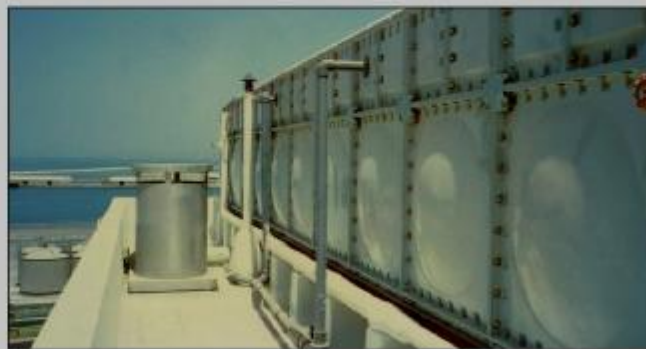
1.5m. Deep, PUF insulated panel tank for drinking water in KSA, with FRP skin for protection of PUF)
