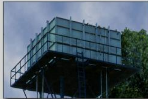
2.5m deep 62.5 KL tank for drinking water at a Railway Colony
